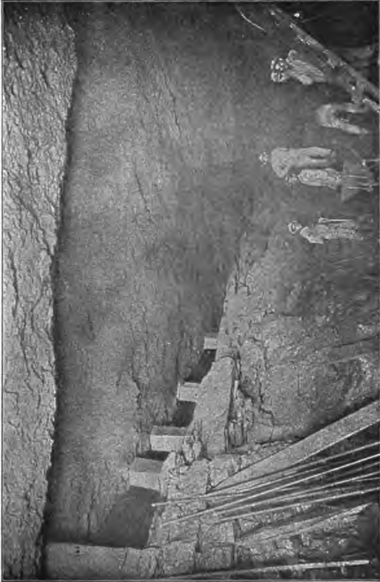
PLATE 89.—Tunneling through Limestone Containing Water-worn Caves Found to be Filled with Clay. Note water-worn roof and clay seam below roof.
